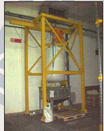
Scarico big bags. Discharge of big bags.
